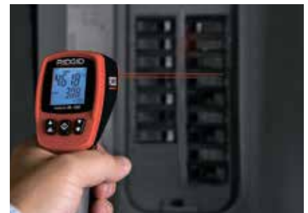
Check fuse or circuit breaker overheating, which could be caused by overloaded circuits
